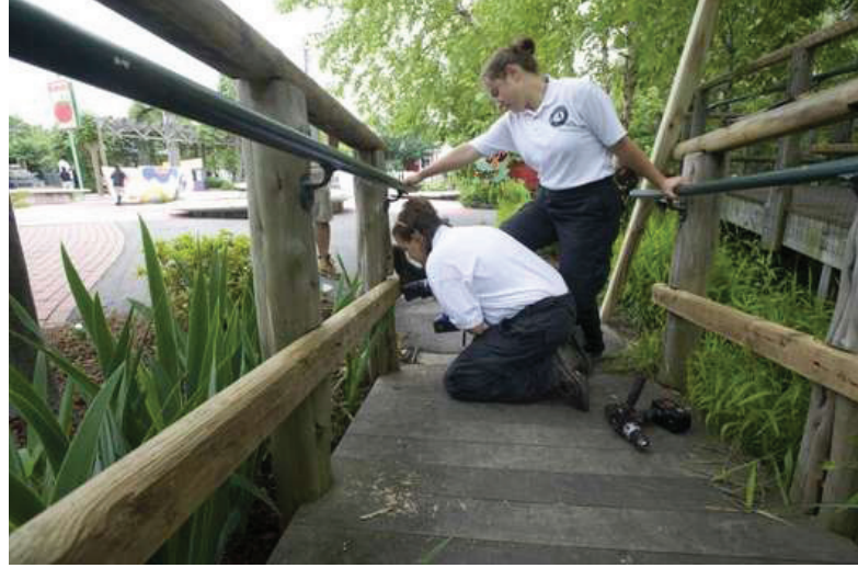
Avi Steinhardt/Courier-Post 6/10/09 -- Americorps volunteers Sadie Stone (left) and Noel DiDomenico replace a fence railing at the Camden Children's Garden.
